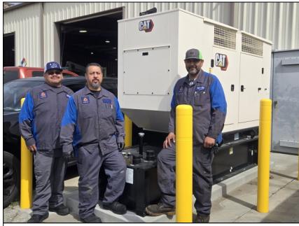
New Tier 3 Generator at Public Works.
