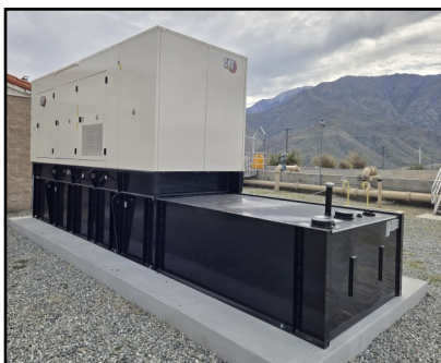
New Tier 3 Generator at Waste Water Treatment Plant.
