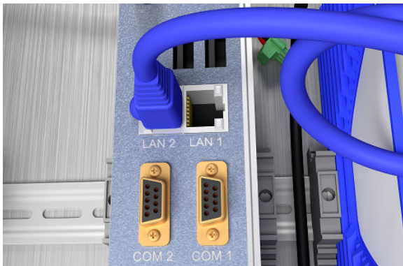
Figure 95. LAN 2 and LAN 1 Ports on the Standard Tesla System Controller
